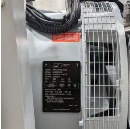
Nameplate on Diesel Generator
