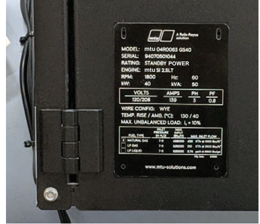
Nameplate on Gas Generator
